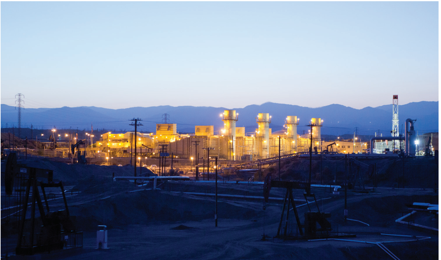
Sycamore cogeneration plant in Kern River. Gas-fired cogeneration facilities are examples of highly efficient energy production, generating electricity from the turbine-powered generator and steam from the turbine exhaust. The electricity is exported to the utility grid, while the steam is used by Chevron for thermally enhanced oil recovery. Each unit can generate up to 75 megawatts of power and 30,000 barrels (cold water equivalent) of steam per day.
